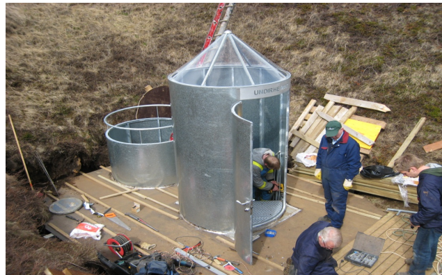
Fig. 9. Work on the platform advances and the cover over the spiral staircase is in place.
